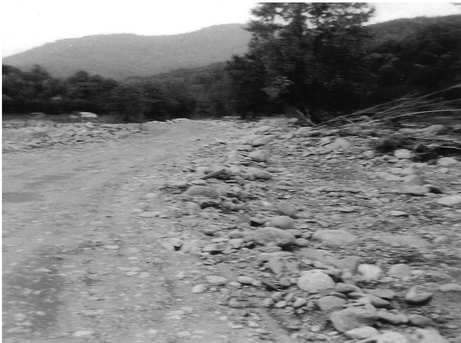
The main road through Tyro washed out, looking west
