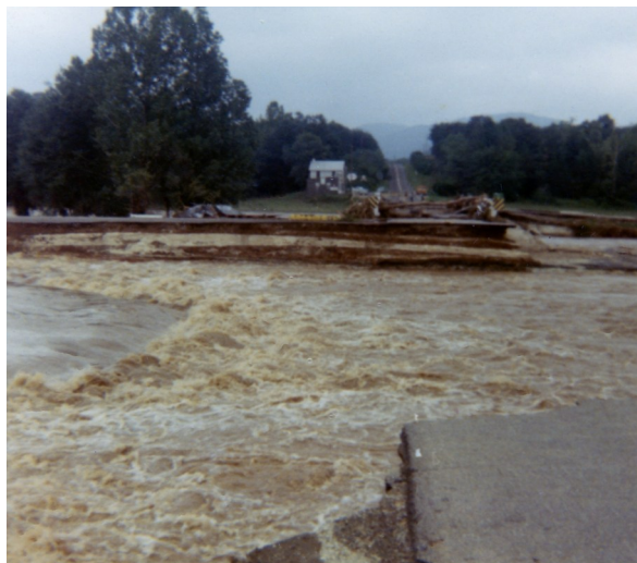
Hwy embankment breach threatens lives near Macs - V Wood _ Lane Ford
